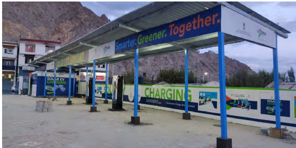
Figure 1- Solar Carport at Leh commissioned by CESL
